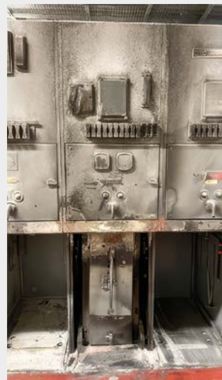
↑ Electrical arcing and fire was caused by failure of GEC VMX high voltage vacuum circuit breaker
