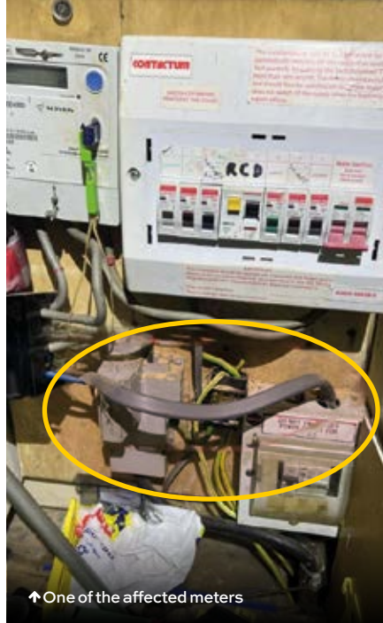
↓ Trying to steal electricity increases the risk of fire
